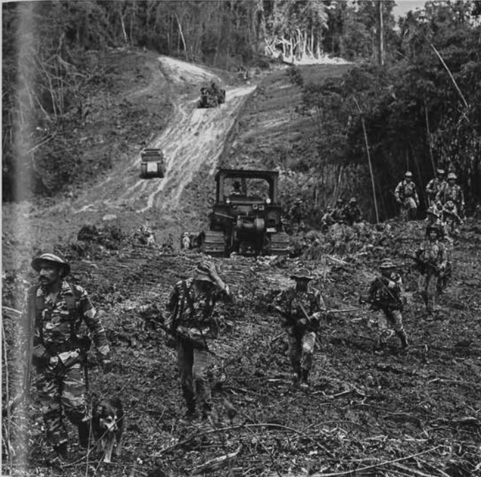
More roads mean fewer guerrillas. Or so believes the Guatemalan Army, which suffers substantial casualties while connecting new towns throughout the rain forest. Treading lightly near the Xacbal River, army road builders diligently guard against ambush and snipers.
